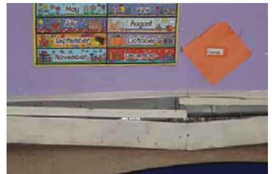
Broken baseboard heating system
