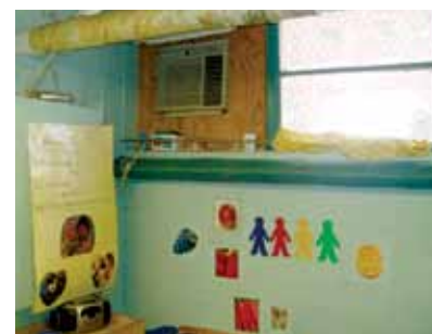
ECE classroom with poor IAQ
